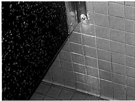
See required corrective action page Line # 8
