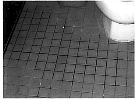
See required corrective action page Line # 9
