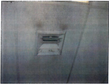
See required corrective action page Line # 46 & 47
