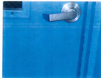
See required corrective action page Line # 17
